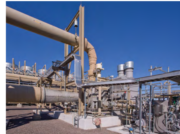
Generating electricity from geothermal heat.
